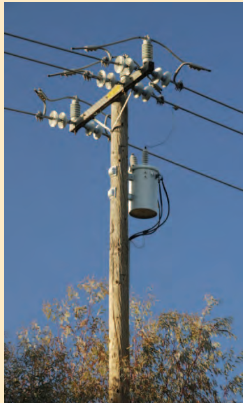
Figure 10.27 A residential utility transformer. (tomba/iStockphoto)
